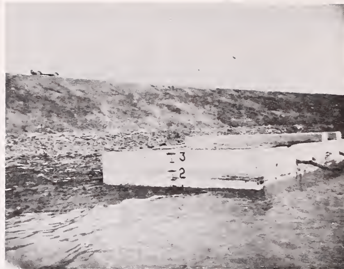
Photo No. 6.—1/29/69 West face of Princ. Splway [principal spillway]. w/s [water surface] appeared to be at indicated 1 9 above crest elevation. 2:30 p.m.
